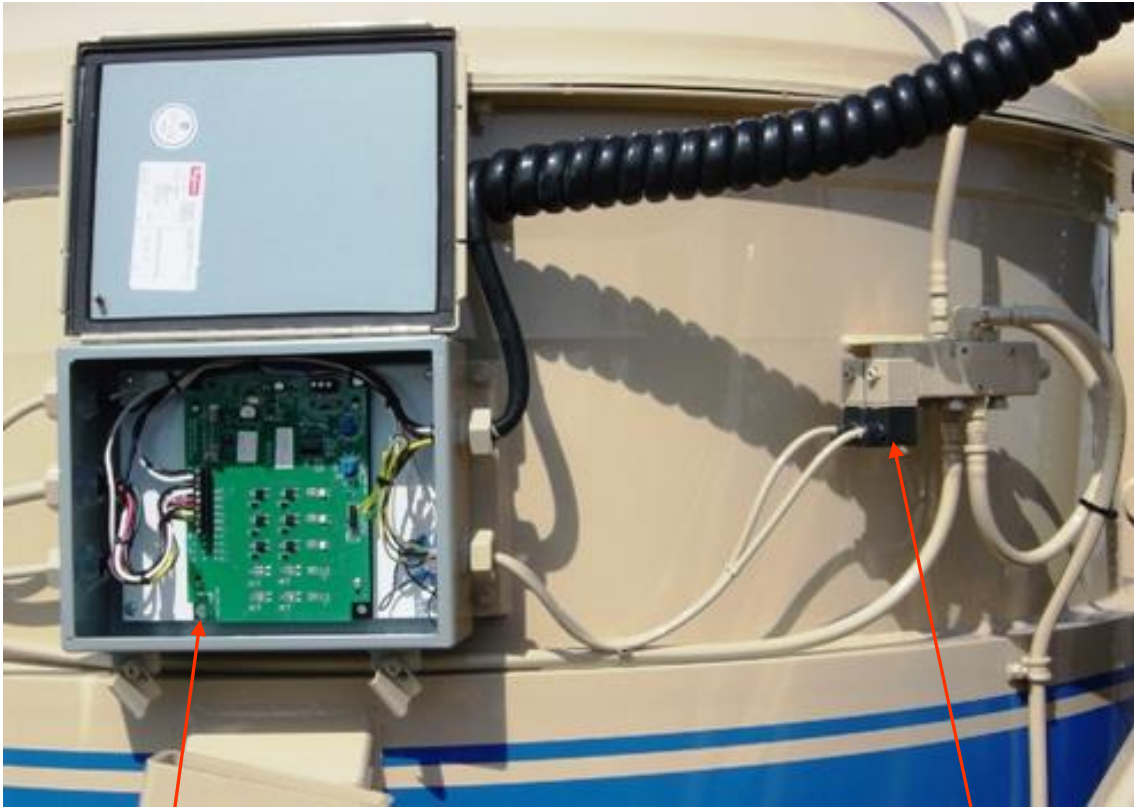
Baghouse Timer Board
